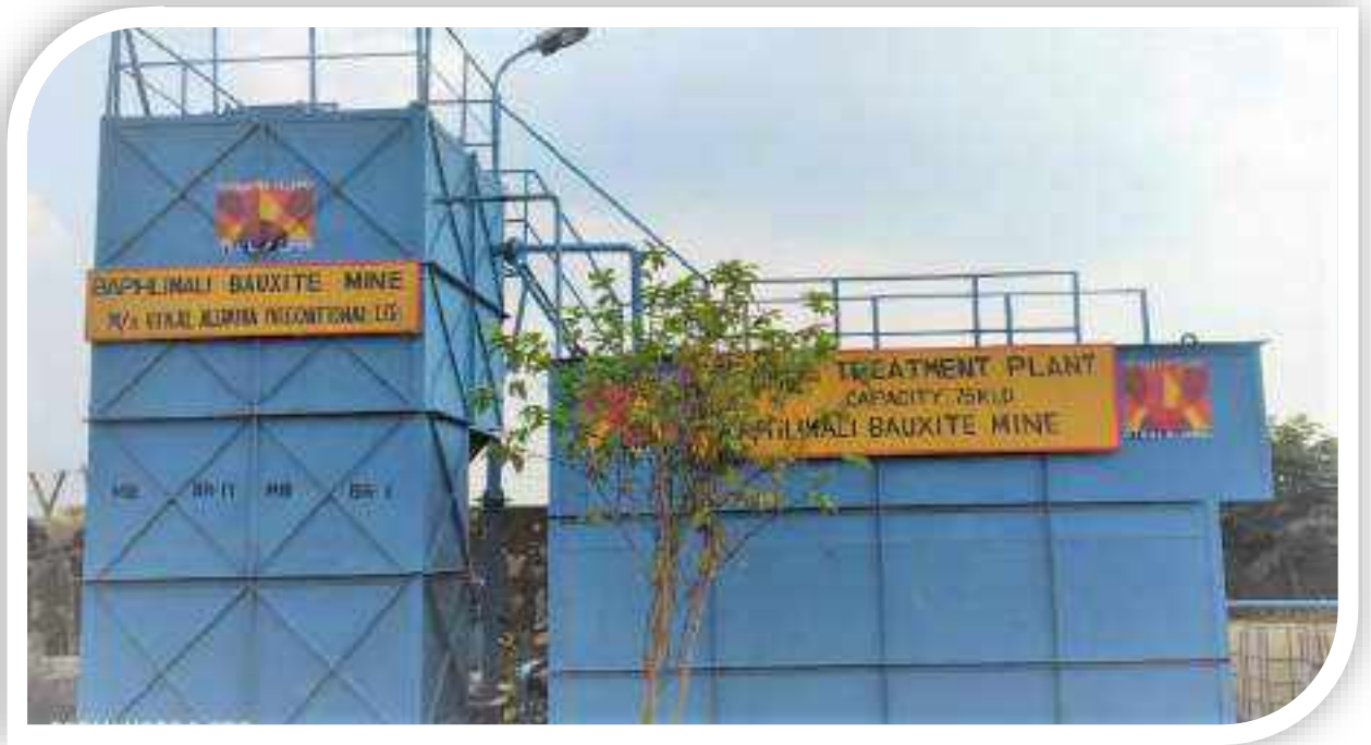
PHOTO 16: Showing 15 KLD Effluent Treatment Plant(ETP)
