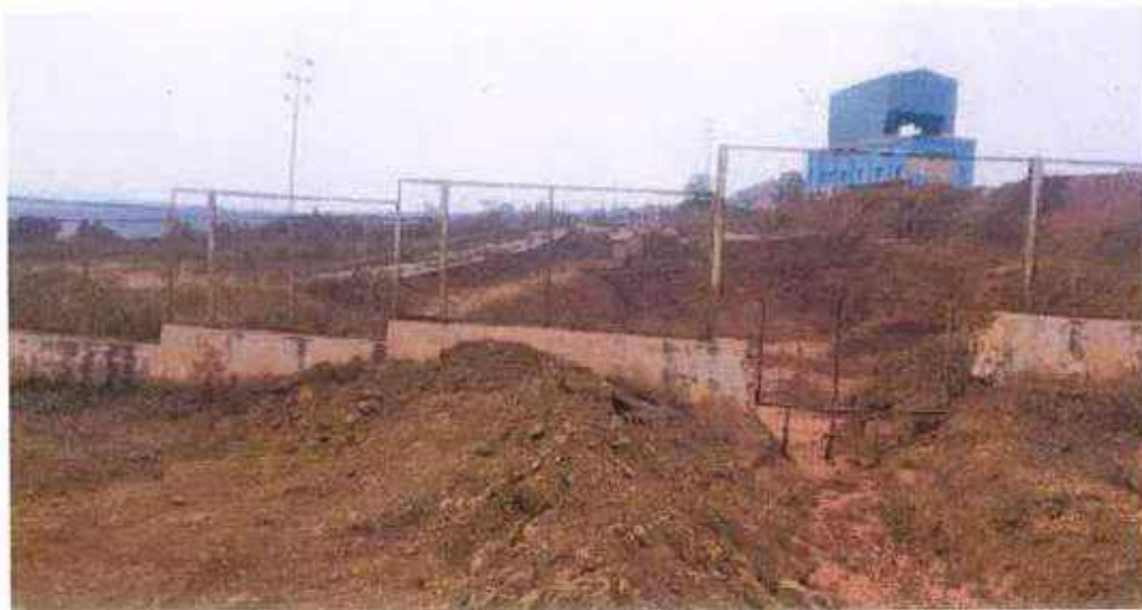
Figure 10: Fencing around the settling pit
