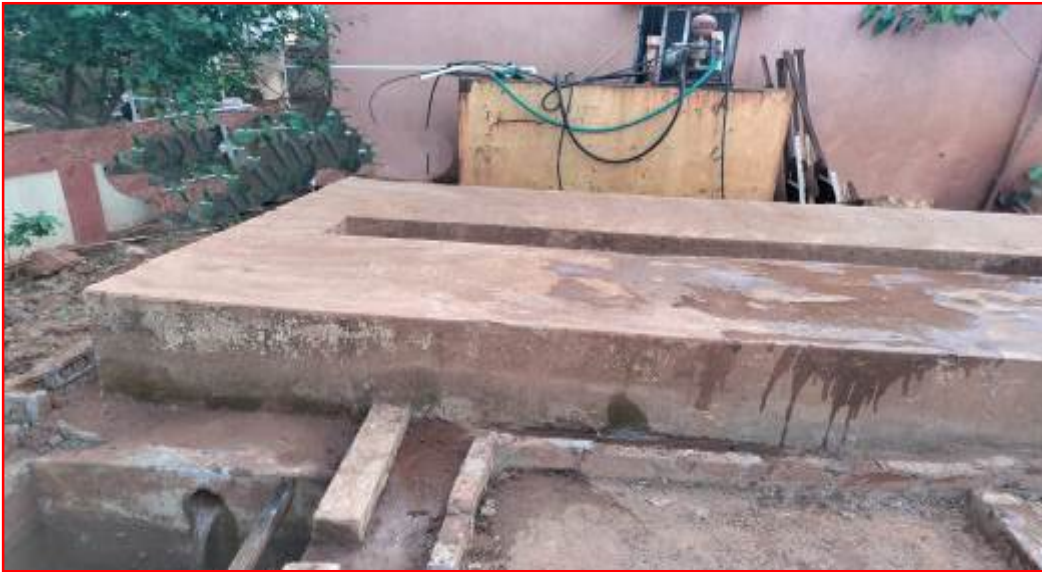
Washing Ramp with Oil and Grease trap
