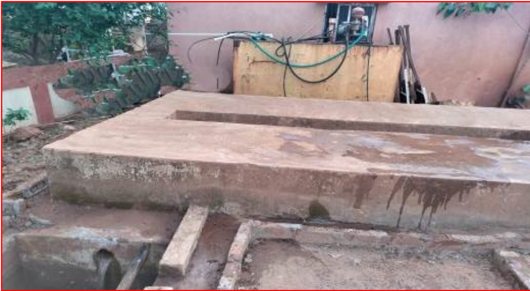
Washing Ramp with Oil and Grease trap
