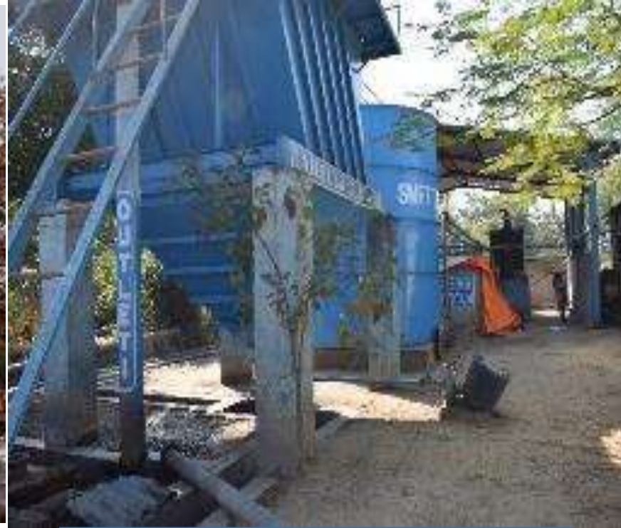
RO Plant for Drinking Water Supply
