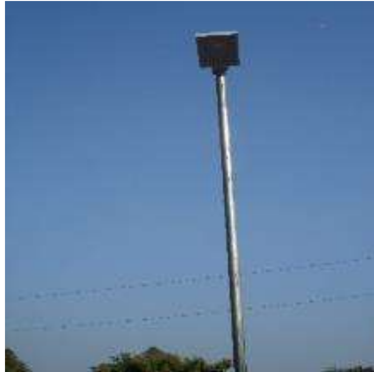
Installed Solar Street Lights
