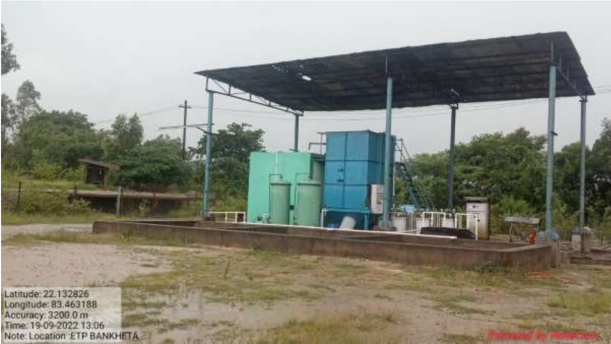
Effluent Treatment Plant – 50 KLD - Bankheta
