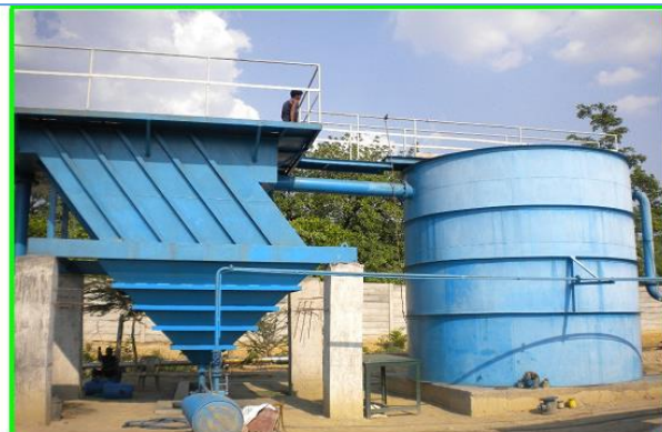
Effluent Treatment Plant - Kondkel – 200 Cum /Hrs X 2
