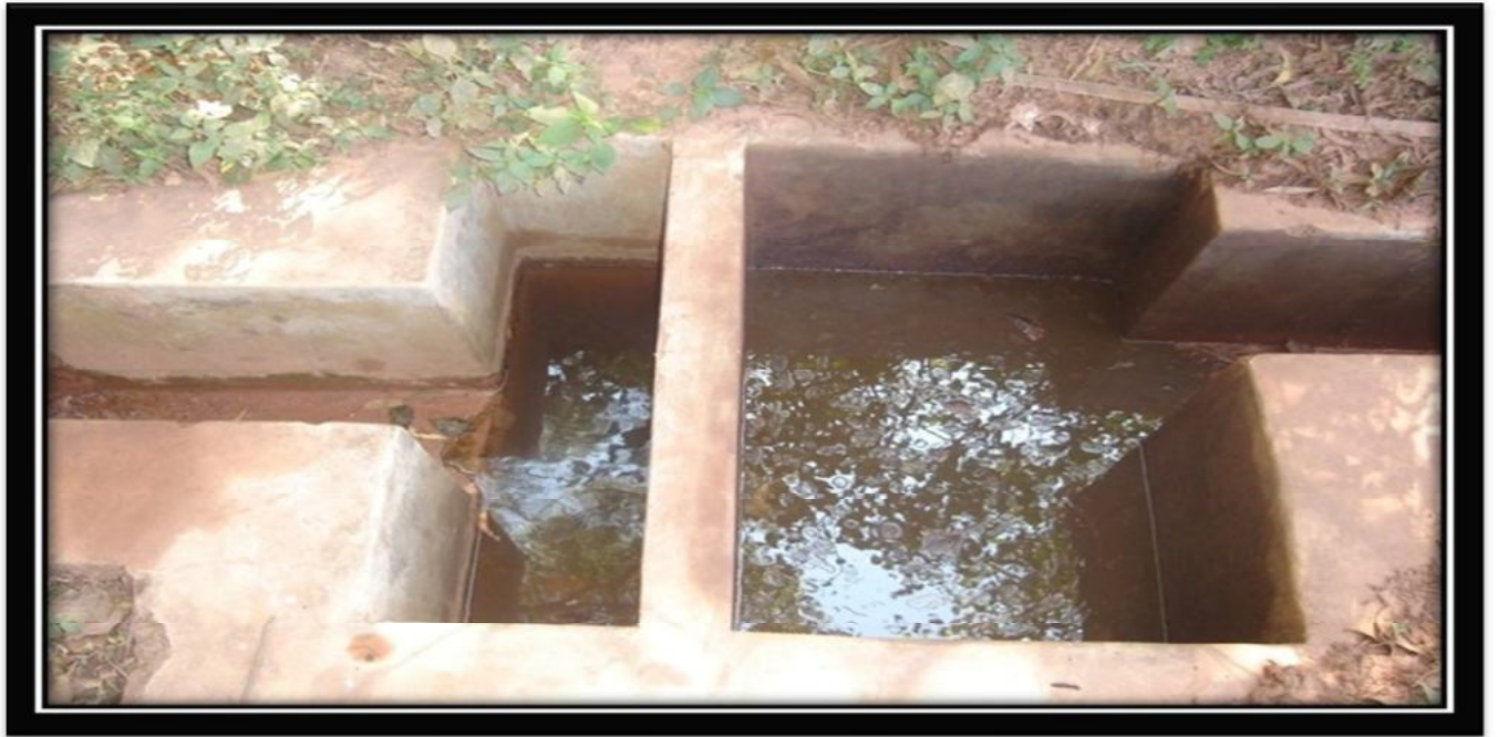
Oil & Grease Trap
