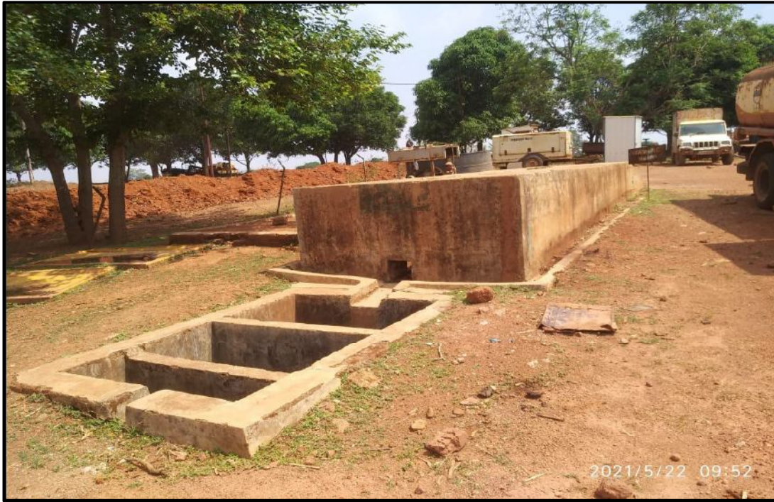
(Washing Ramp and Oil and grease trap)
