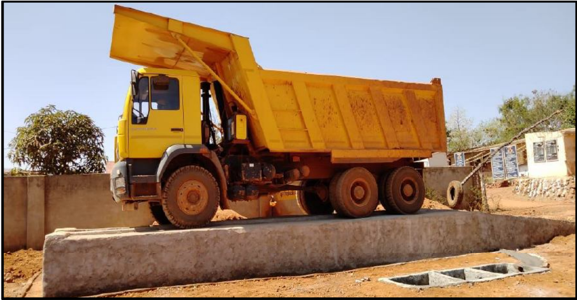
(Pic: Washing platform and oil & grease trap)
