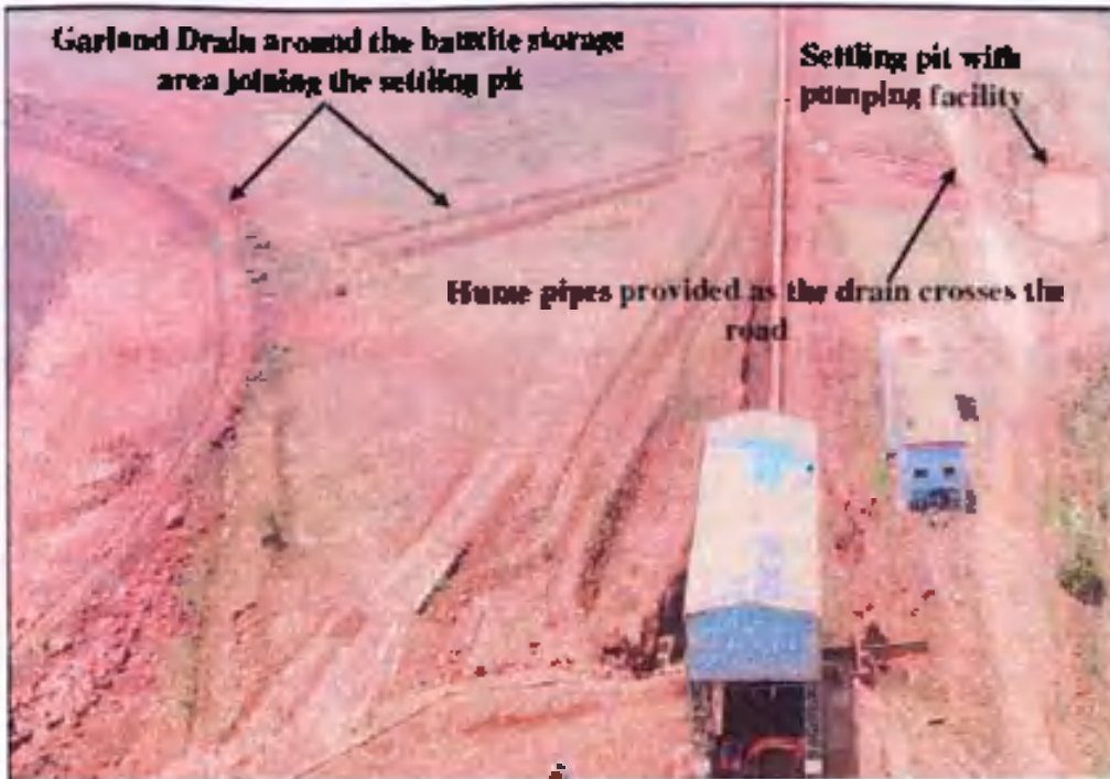
Figure 5: View of earthen retaining wall and garland drains near the bauxite storage area and crusher
