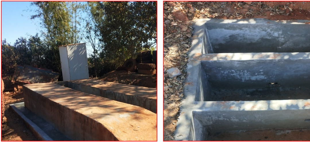
Oil And Grease Trap at Mines
