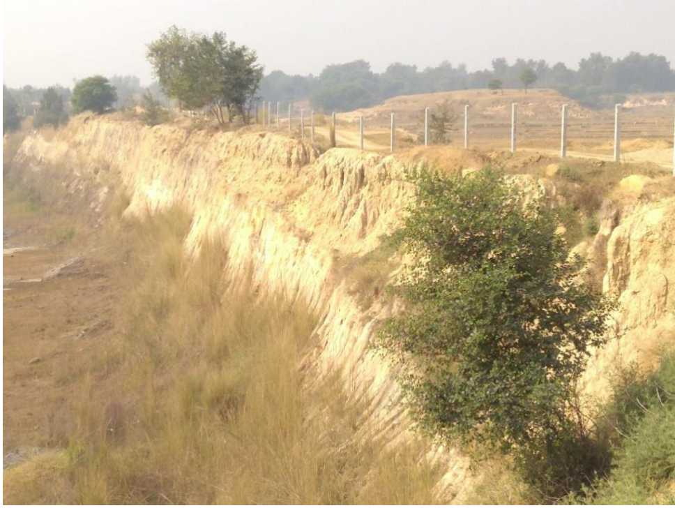
Figure 4: Embankment was on the mine site as seen from the northern end. Erosion of the wall is clearly visible.
