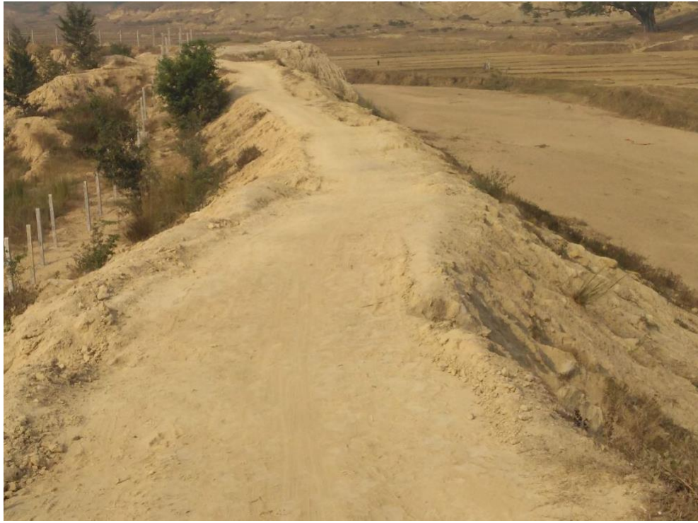
Figure 2: General view of the embankment top from the northern end, visible on the right is the dry river bed
