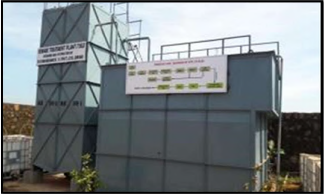
PHOTO 14: Showing 75 KLD STP
