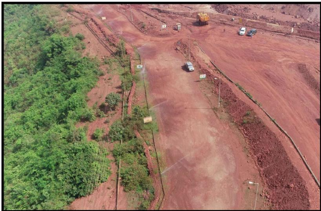
PHOTO 9: Showing Fixed Sprinklers
