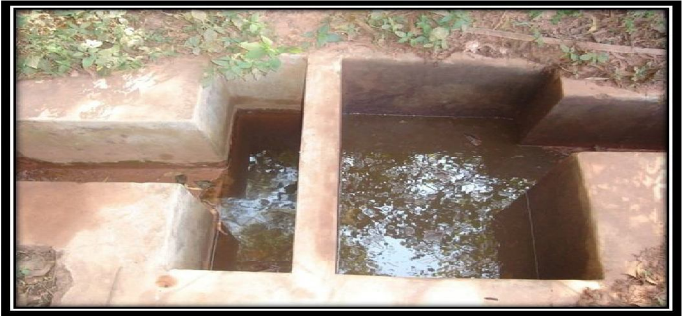
(Oil & Grease Trap)
