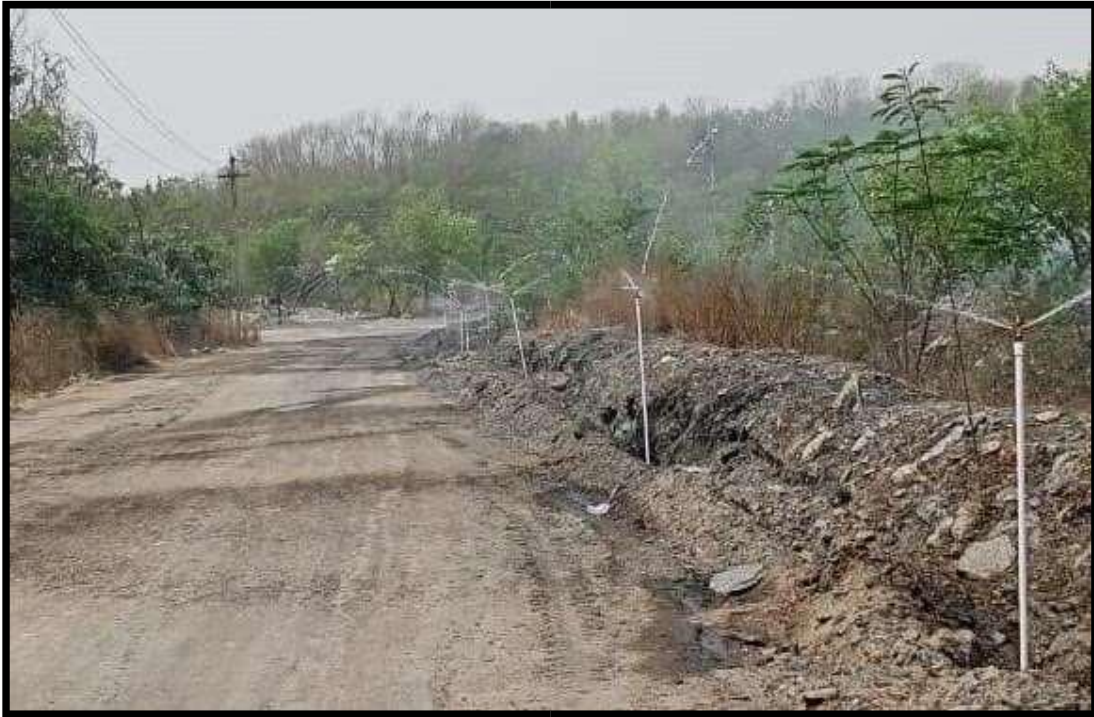
Fig 06- Fixed Type Water Sprinkler along Haul Road
