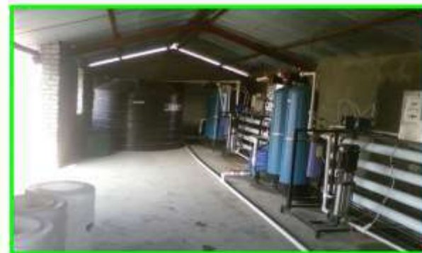
Reverse Osmosis Plant (RO Plant) - Kondkel 2 x 2 Cum/Hrs
