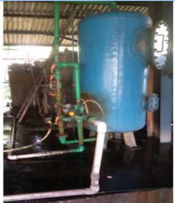
Iron Removal Plant (IRP Plant) – Milupara – 5 Cum / Hrs.
