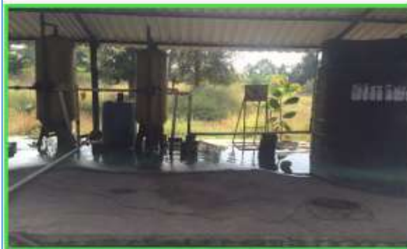
Water Treatment Plant (WTP) - Kondkel - 5 X 5 Cum / Hrs
