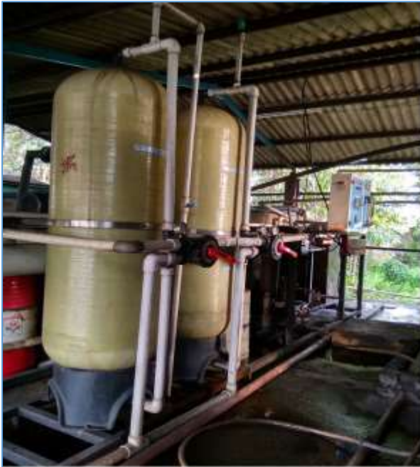
Reverse Osmosis Plant (RO Plant) – Milupara – 5 Cum / Hrs.
