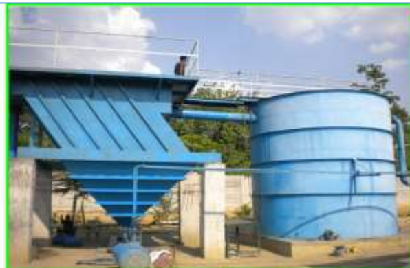
Effluent Treatment Plant - Kondkel - 200 Cum /Hrs X 2
