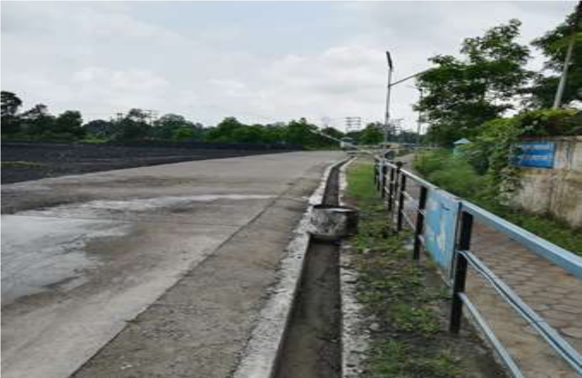
Fixed type of water sprinklers GP IV/5 coal mine
