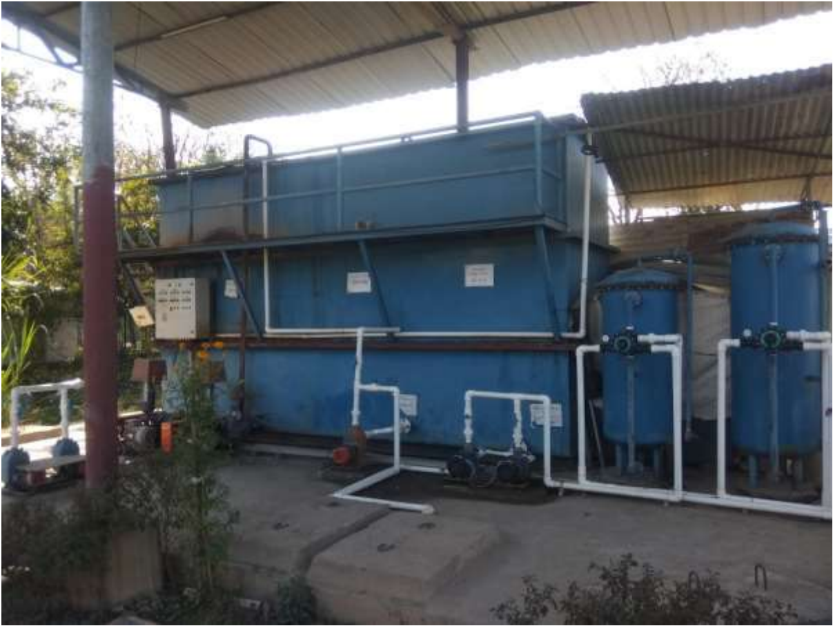
Sewage Treatment Plant – 50 KLD
