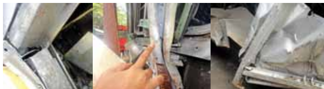
Resulting in Failures at Joints
