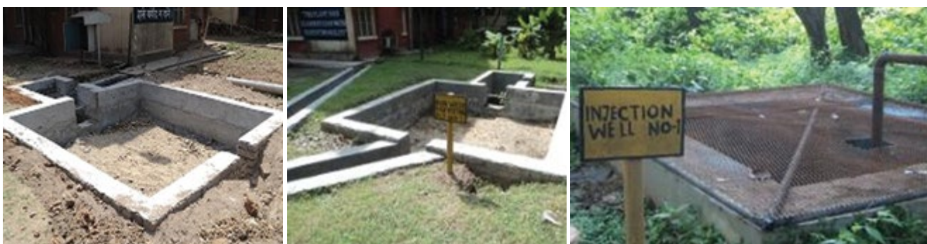
Rain Water Harvesting Units
