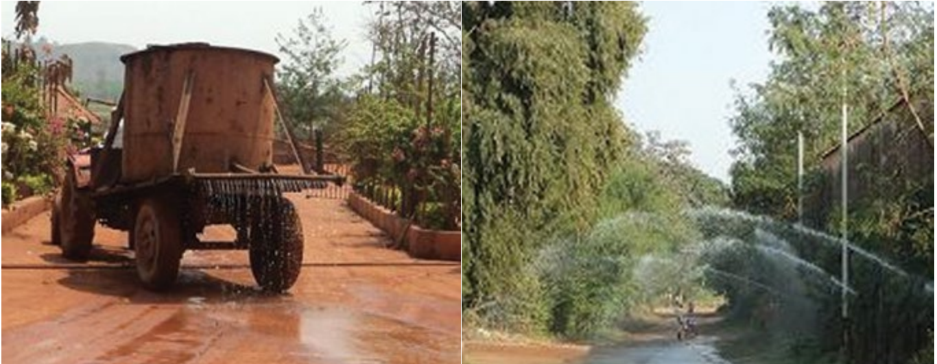
Dust Suppression System by Using STP treated water
