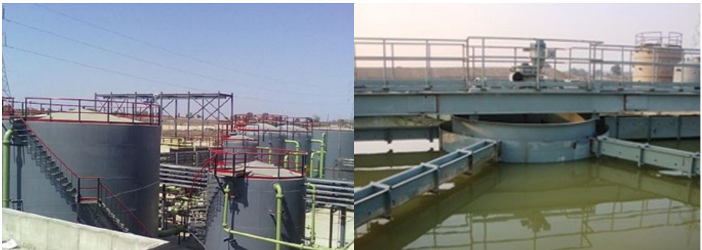
Recycling of waste water by effluent treatment in Mahan Plant
