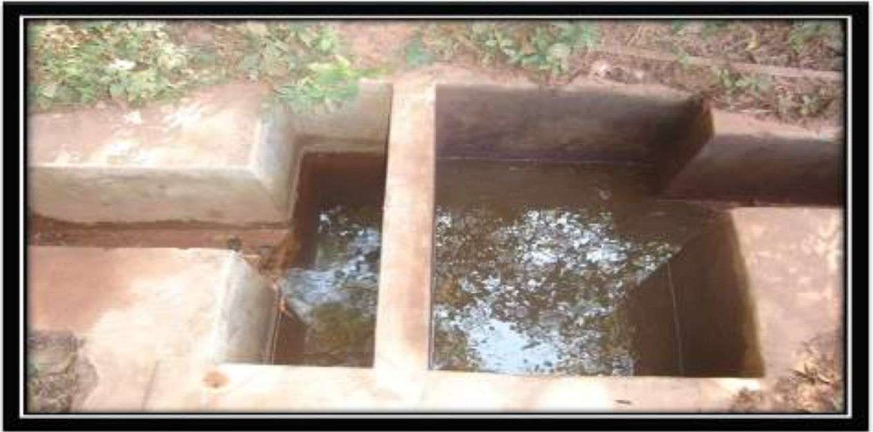
Oil & Grease Trap
