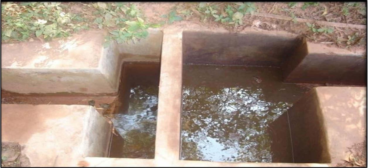
Oil & Grease Trap
