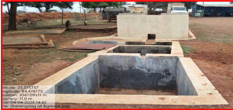
Oil & Grease trap
