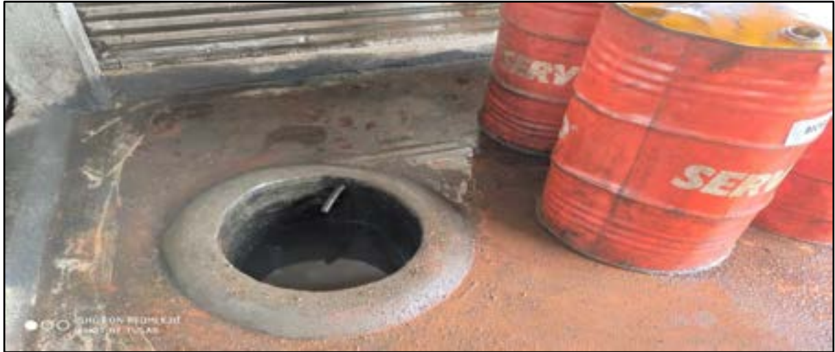
Photographs of Oil and Grease Trap
