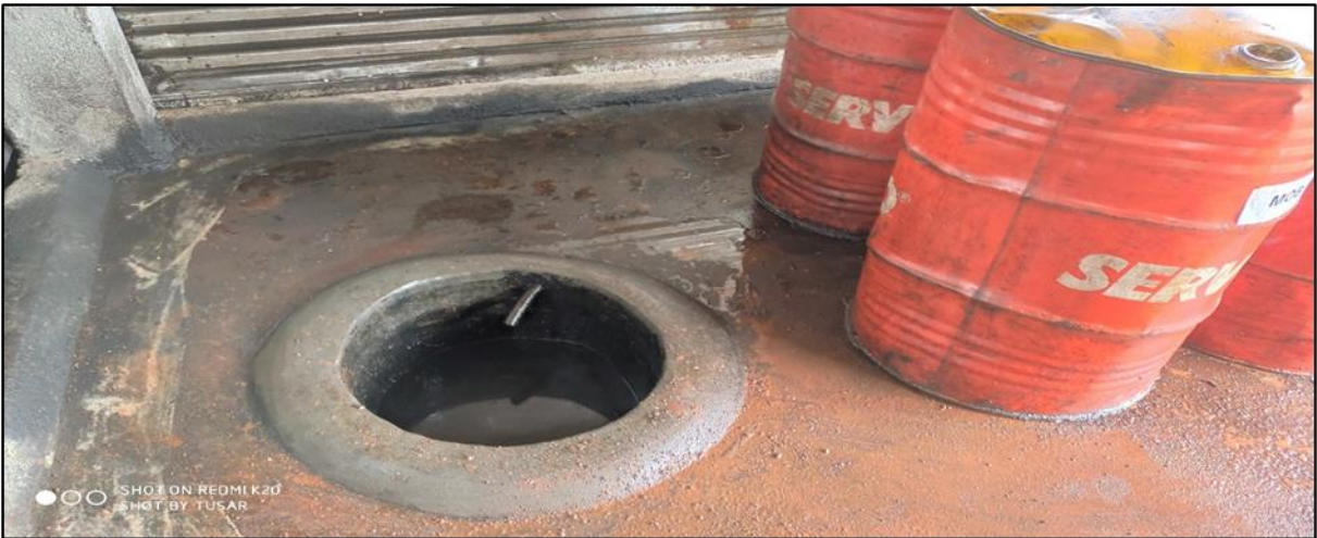
Photographs of Oil and Grease Trap
