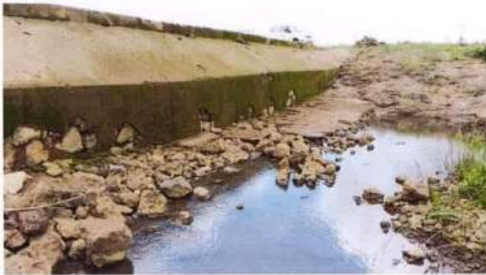
Figure 9a: Photographic view of damaged check dam during 2016
