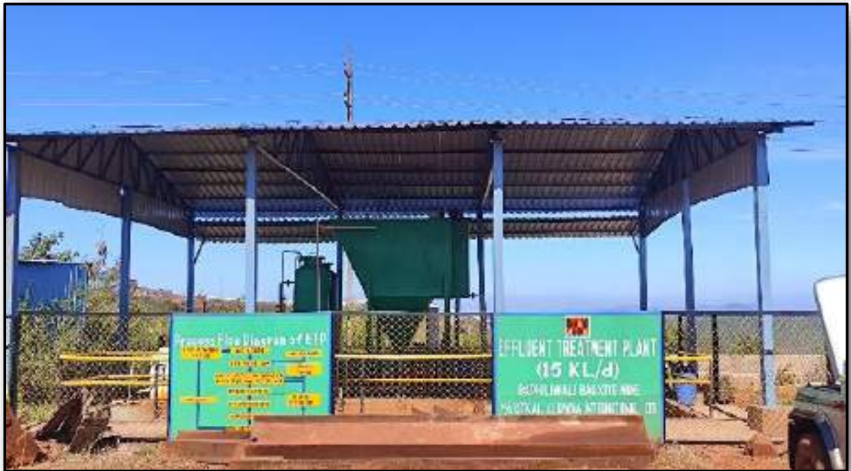
PHOTO 16: Showing 15 KLD Effluent Treatment Plant(ETP)
