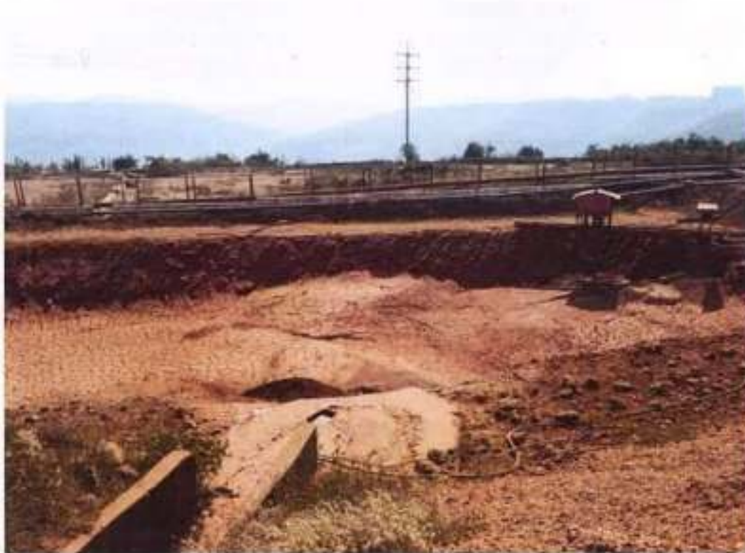
Figure 1: View of settling pit and pumps near the crusher
