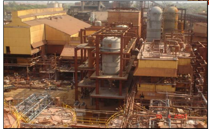
LT digester flash tanks
