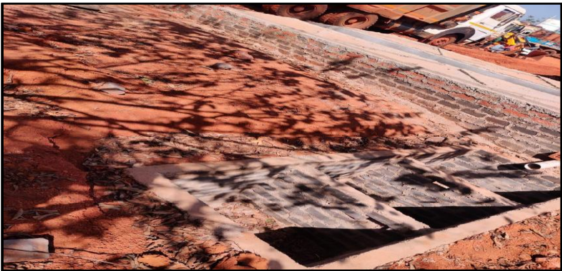
(Washing Ramp and oil-grease trap)
