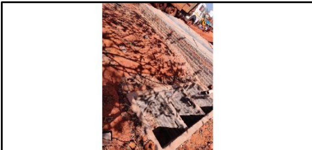
(Washing Ramp and oil-grease trap)
