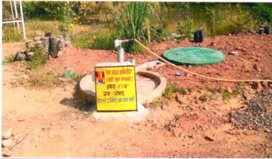
A View of recharge well and Rain water harvesting pond
