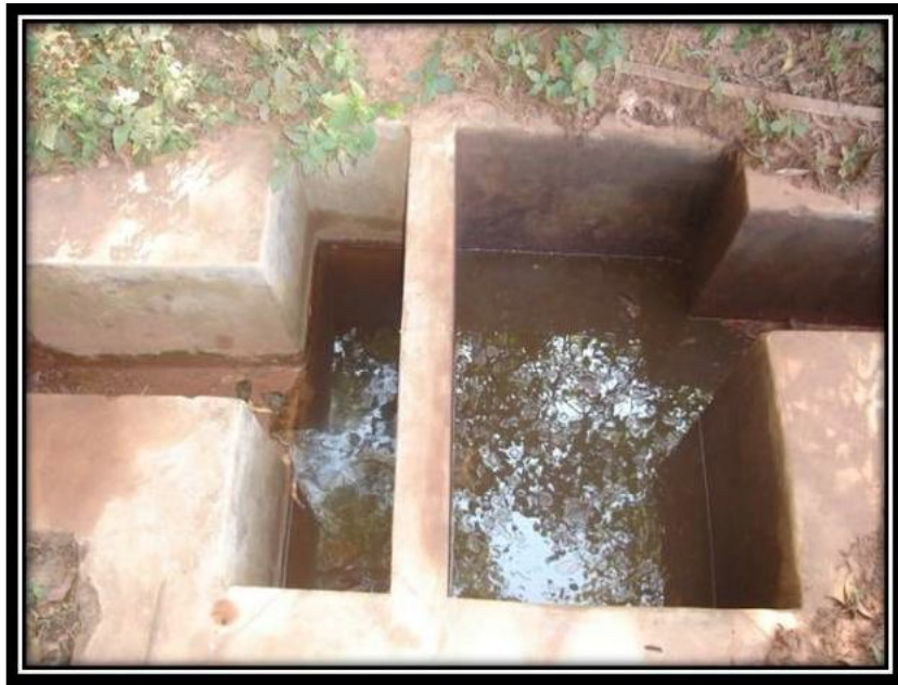
(Oil & Grease Trap)
