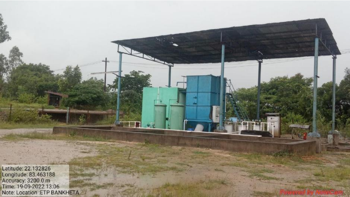
Effluent Treatment Plant – 50 KLD - Bankheta
