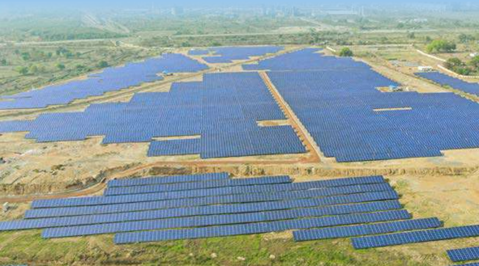
A view of our solar plant at Aditya
