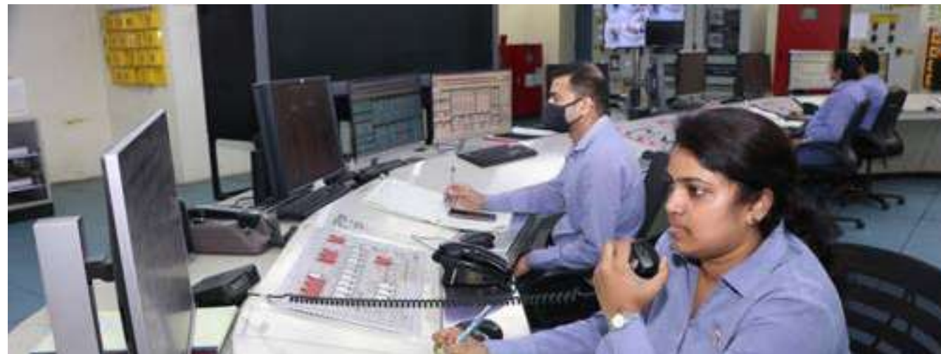
Power plant control room
