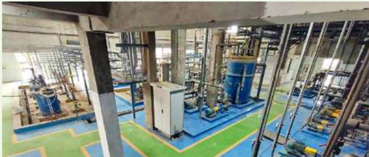
TWRU Pump house
