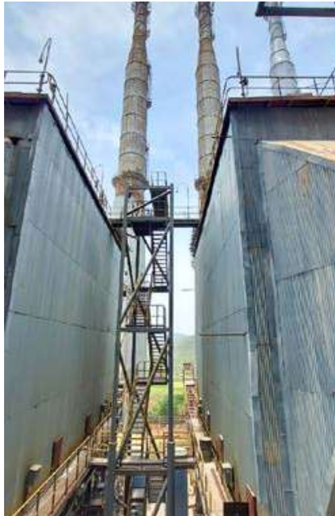
Calciner stack and ESP at Utkal Alumina
