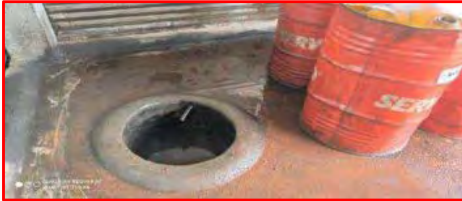
Oil & Grease Trap
