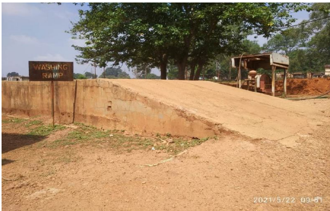
(Washing platform and oil & grease trap)
