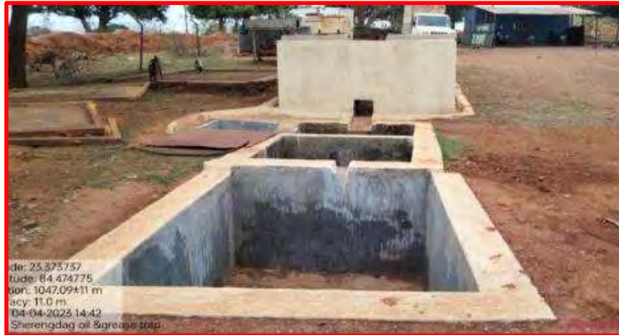
Washing Ramp and Oil and Grease Trap
