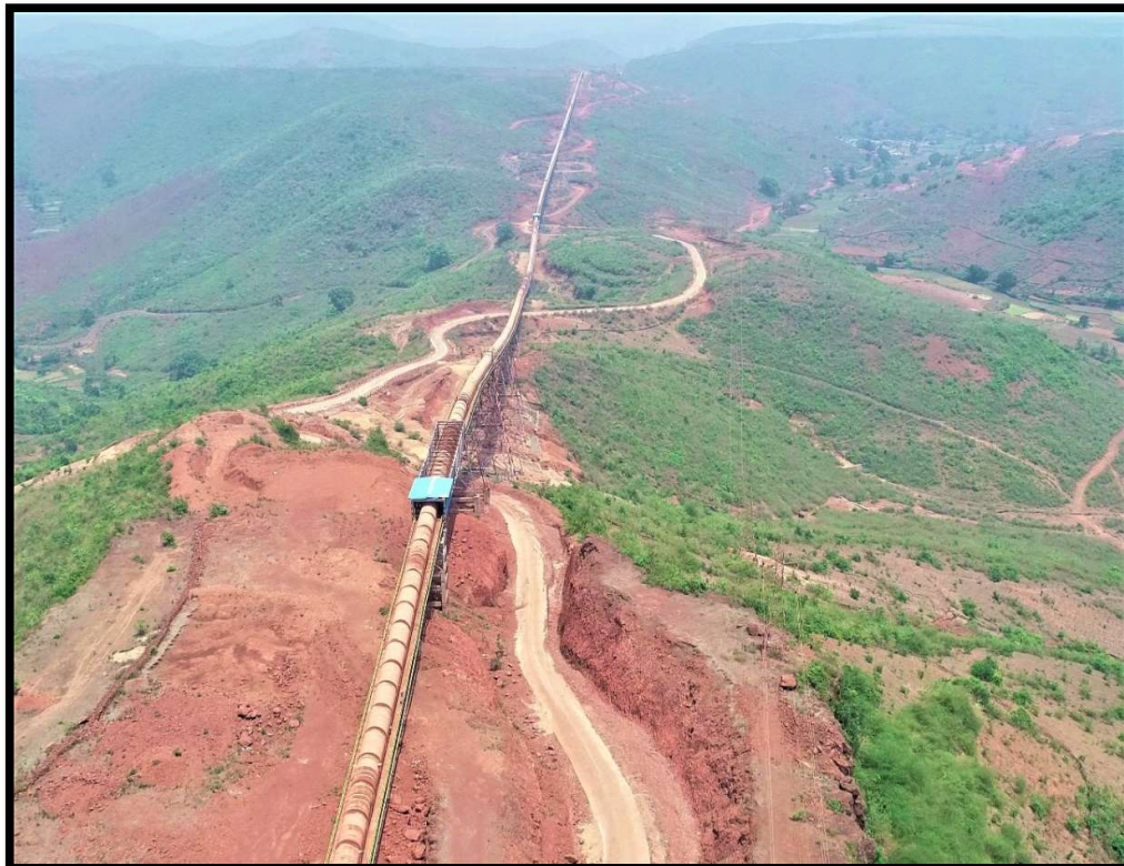
PHOTO 13: Showing Covered Long distance Conveyor
