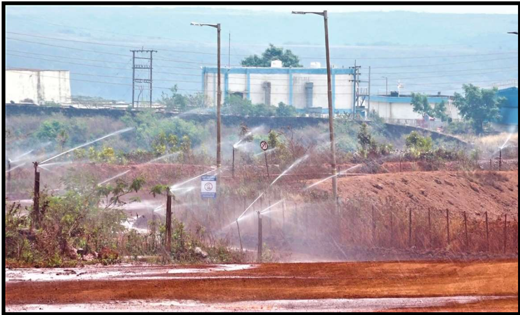
PHOTO 9: Showing Fixed Sprinklers
