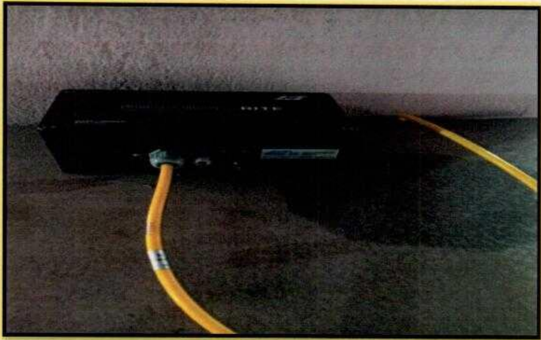
Piezometer Installed in Lease area for keeping a note on Ground water Level
