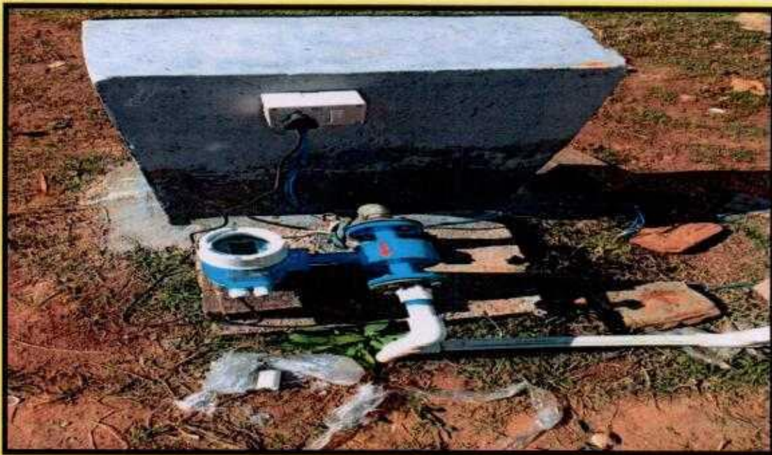
Water Meter installed in Samri Lease to Monitor Water Consumption
