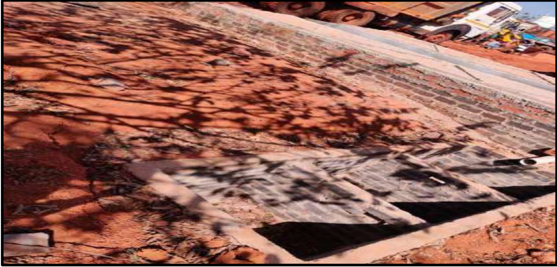
(Washing Ramp and oil-grease trap)
