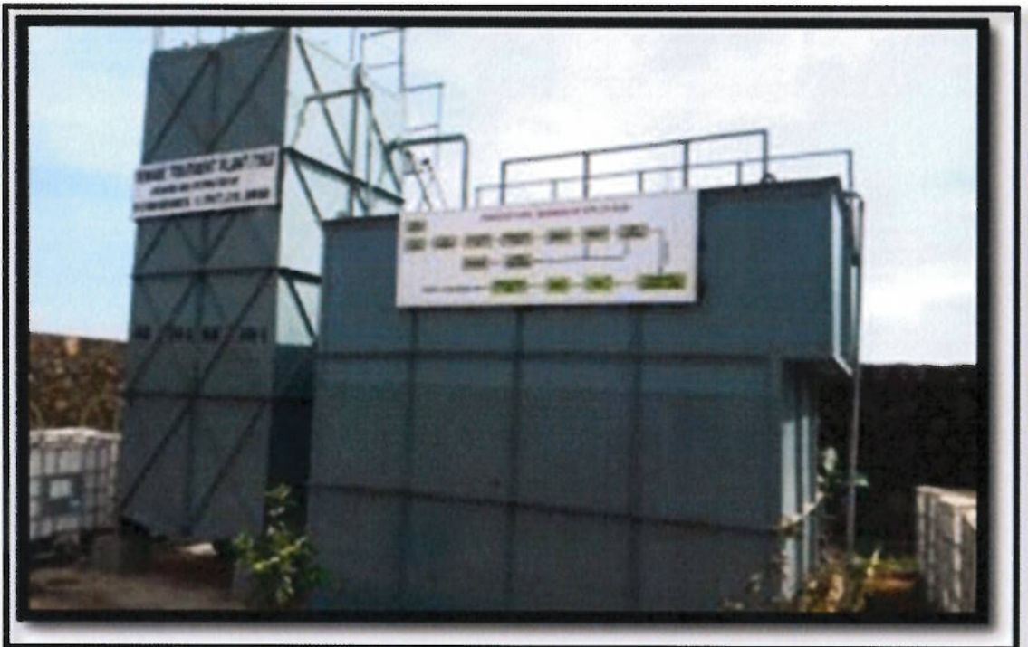
Photo -12 : Showing 75 KLD STP
