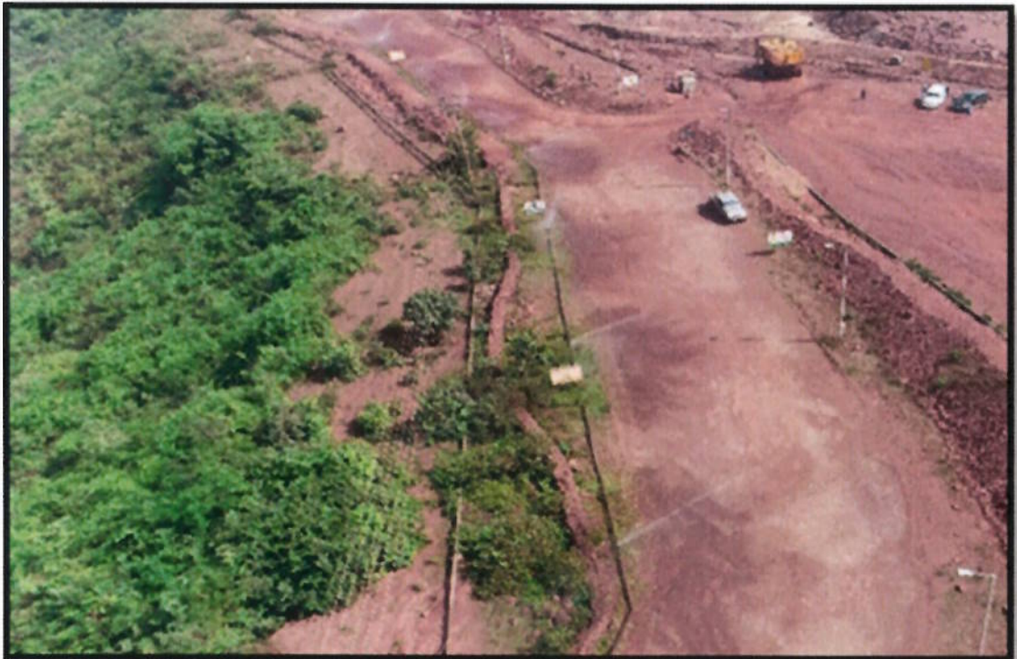
Photo -8 : Showing Fixed water sprinklers in operation
