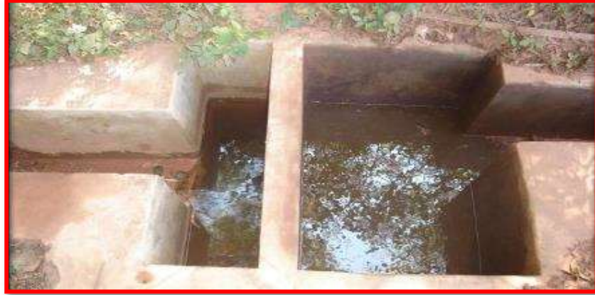
Oil & Grease trap
