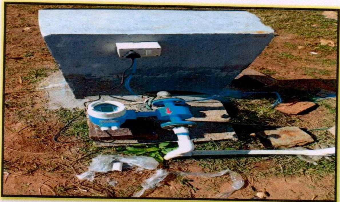
Water Meter installed in Samri Lease to Monitor Water Consumption
