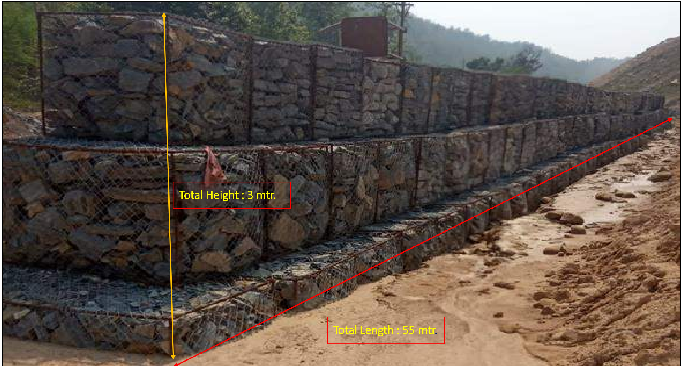
Gabion/Retaining wall at the toe of permanent dump slope for arresting the silt near Patch "C" in Banjikhoh, GP IV/4 Coal Mines.
