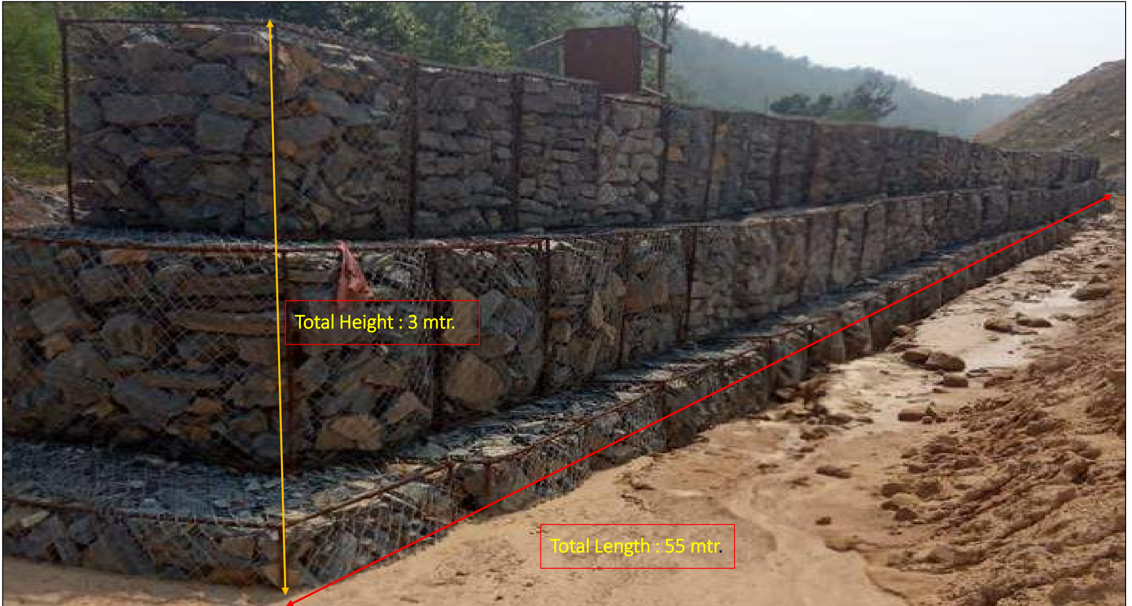
Gabion/Retaining wall at the toe of permanent dump slope for arresting the silt near Patch "C" in Banjikhoh, GP IV/4 Coal Mines.
