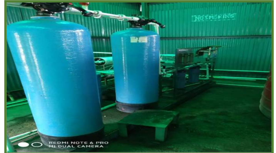
Drinking Water Section (RO Plant 2 KL/Hour)
