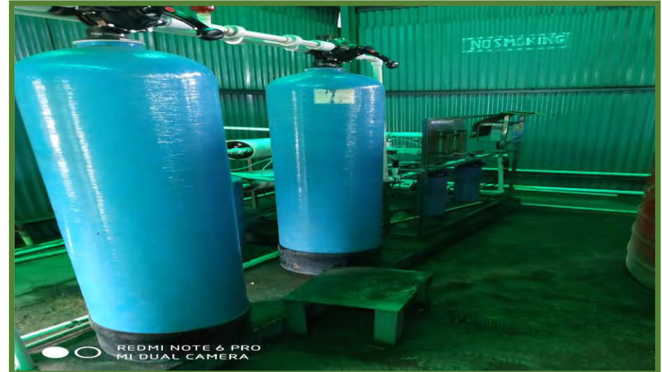
Drinking Water Section (RO Plant 2 KL/Hour)
