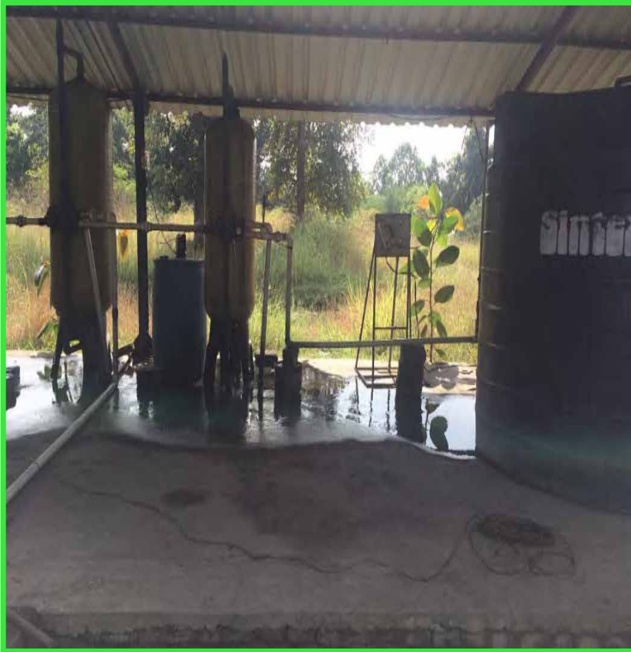
Water Treatment Plant (WTP) – Kondkel – 5 X 5 Cum / Hrs
