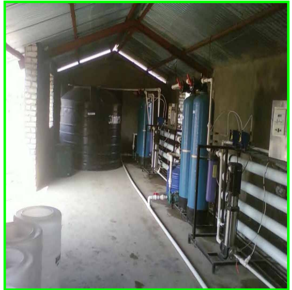
Reverse Osmosis Plant (RO Plant) – Kondkel 2 x 2 Cum/Hrs
