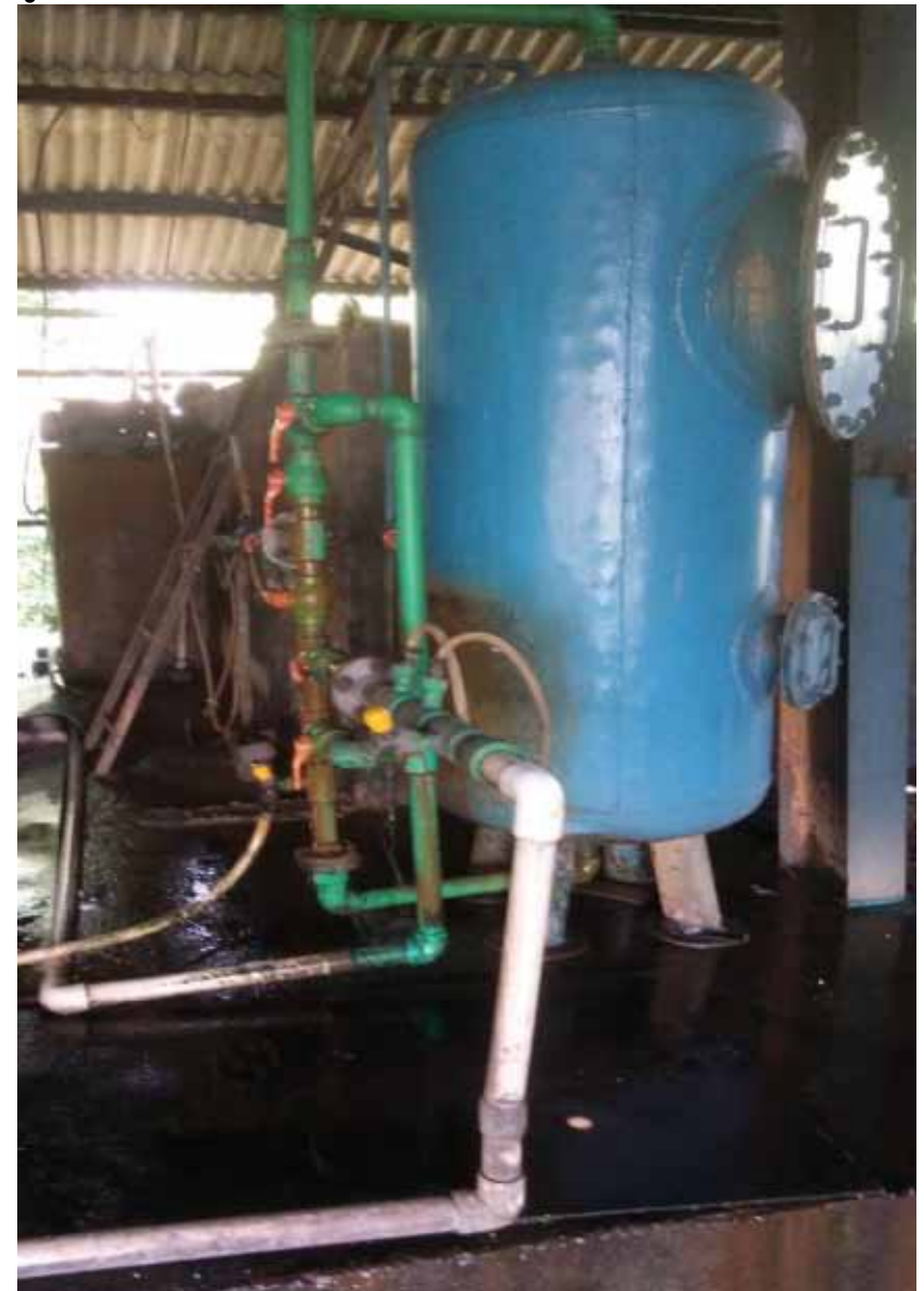
Iron Removal Plant (IRP Plant) – Milupara – 5 Cum / Hrs
