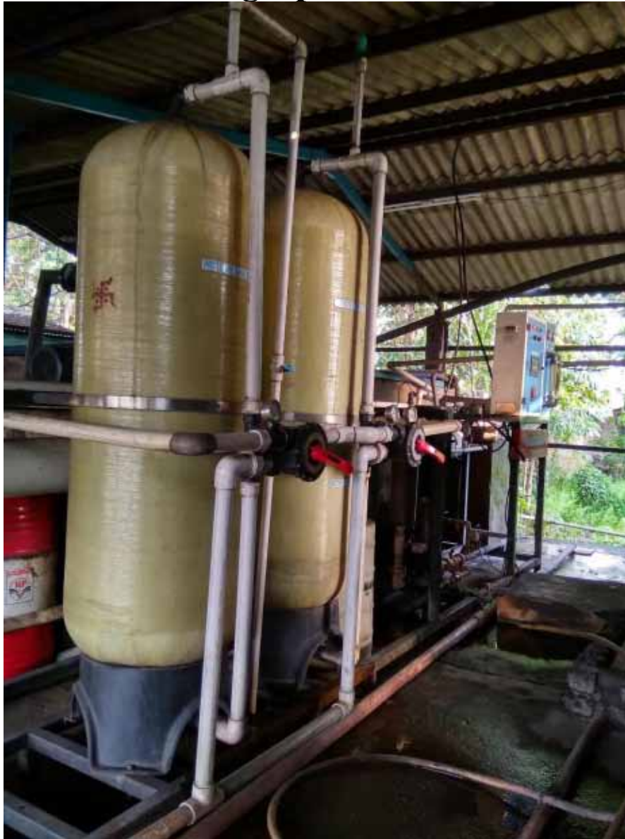
Reverse Osmosis Plant (RO Plant) – Milupara – 5 Cum / Hrs
