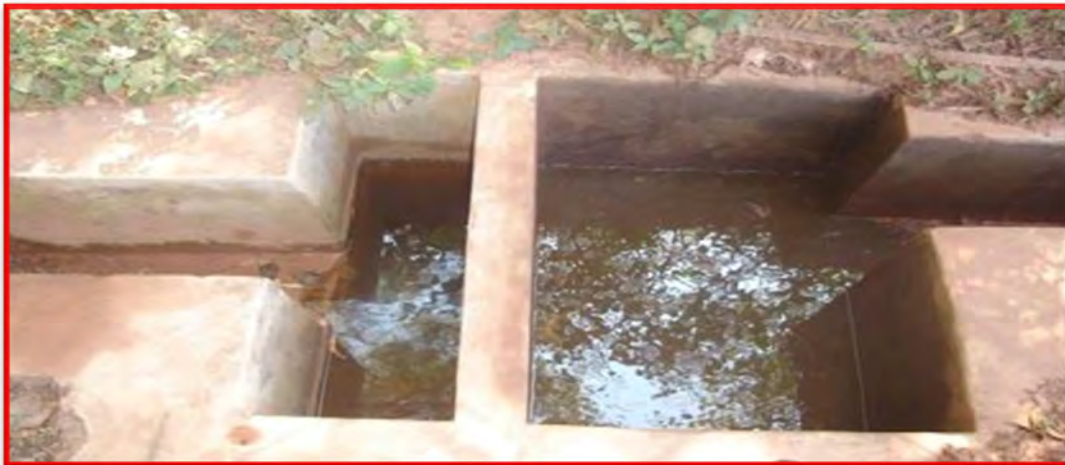
Oil and grease trap
