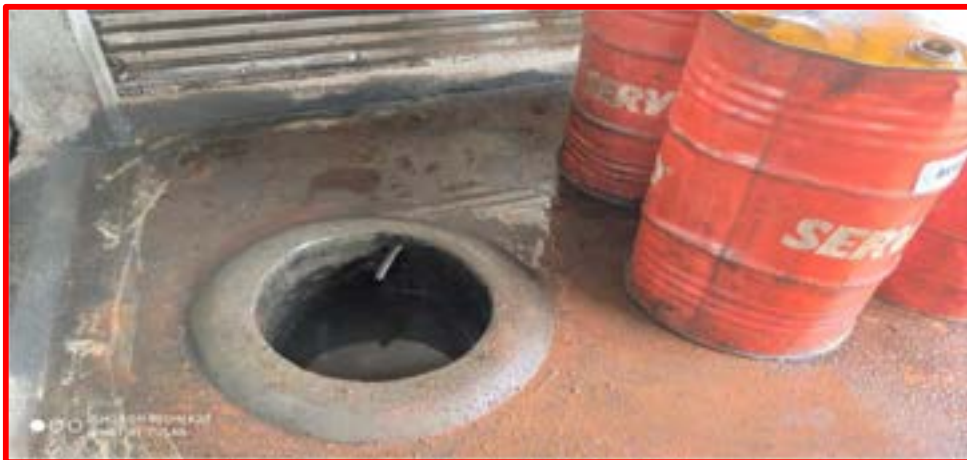
Oil and Grease Trap
