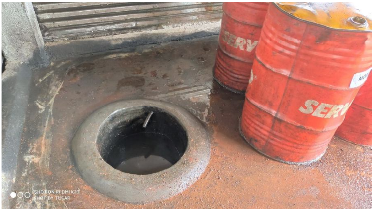
Photographs of Oil and Grease Trap
