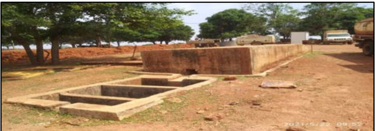
Washing Ramp and Oil and grease trap
