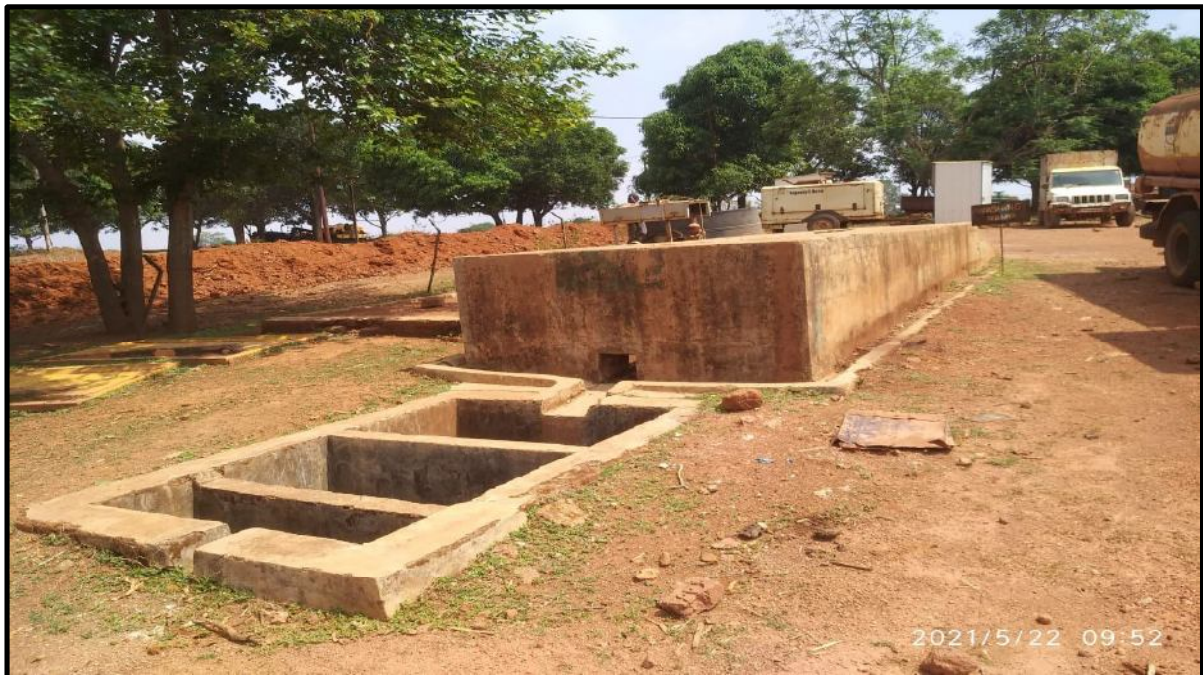
(Washing platform and oil & grease trap)
