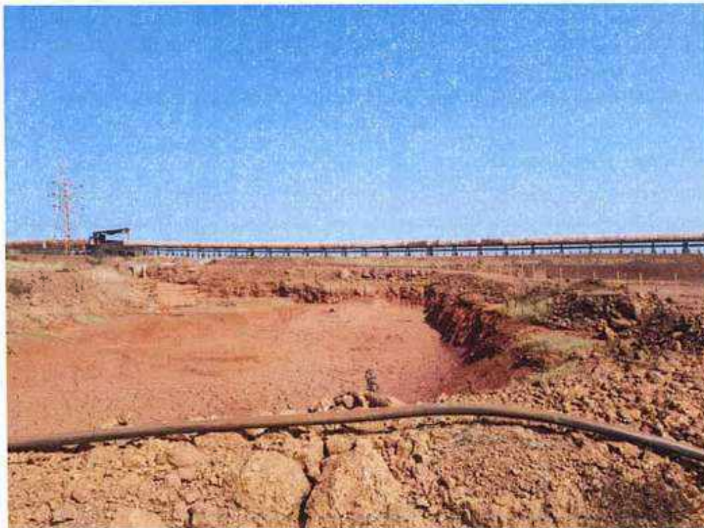
Figure 3: View of the newly constructed 2 nd settling pit near the mine entrance
