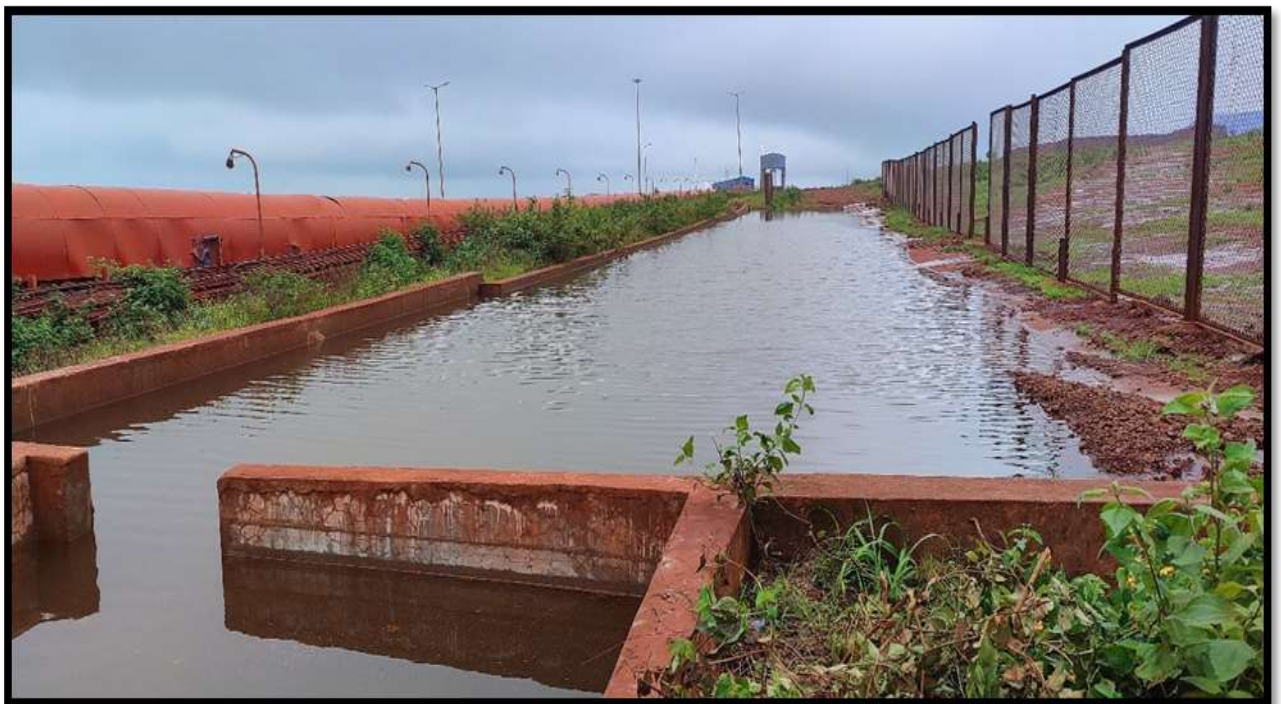
PHOTO 11: Surface Rainwater Harvesting Structure.
