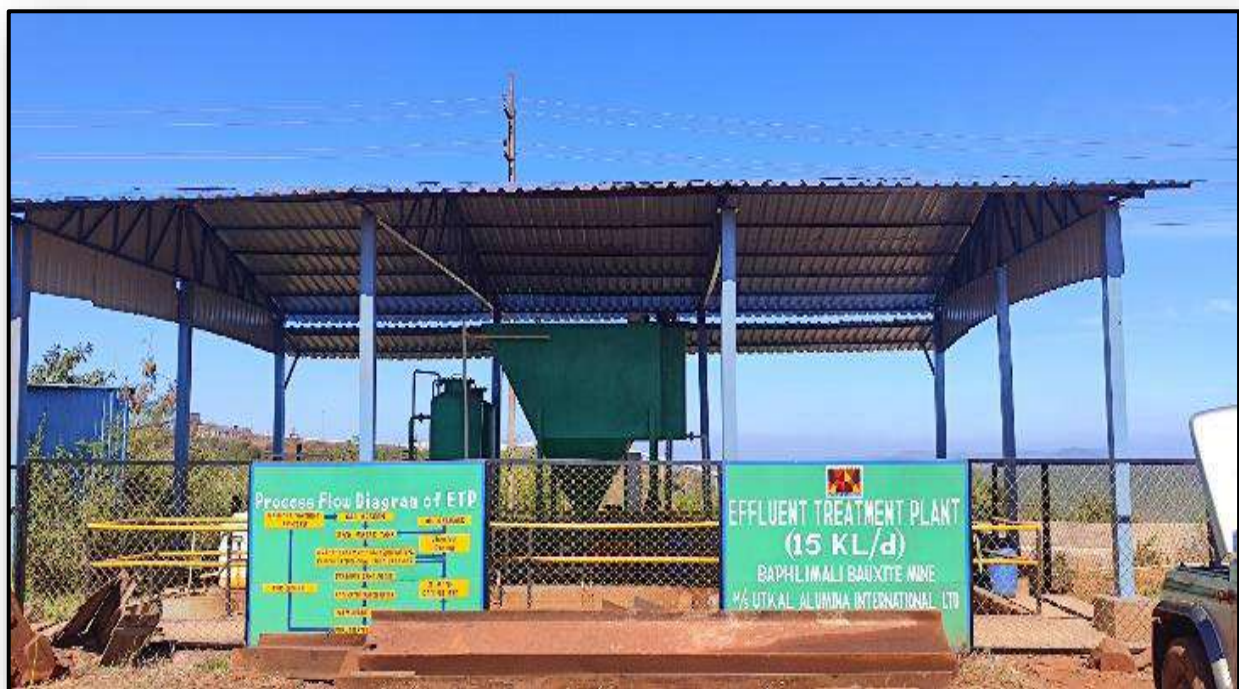
PHOTO 17: Showing 15 KLD Effluent Treatment Plant (ETP)
