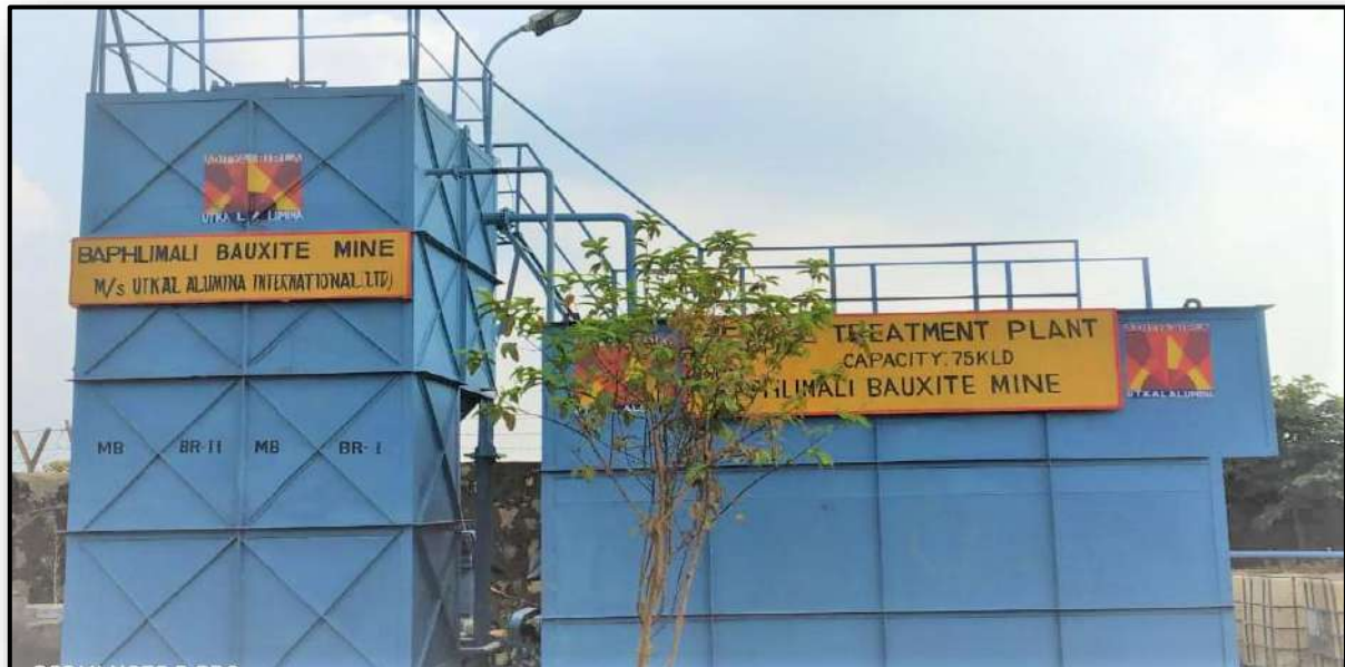
PHOTO 16: Showing 75 KLD Sewage Treatment Plant (STP)
