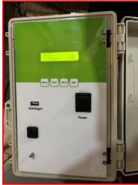
Piezometer Installed at Mine
