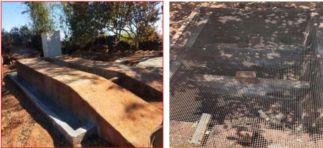
Oil and Grease Trap at Mines
