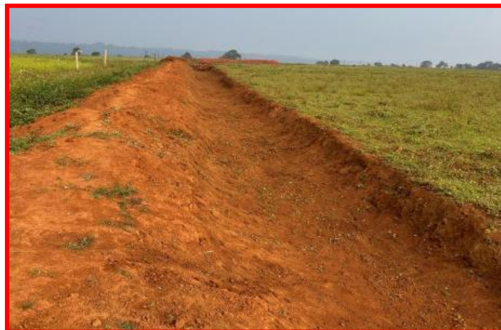
Garland drains around
